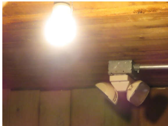
Typical Emergency Light
