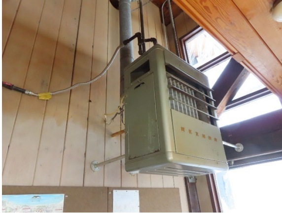
Hanging Reznor Furnace
