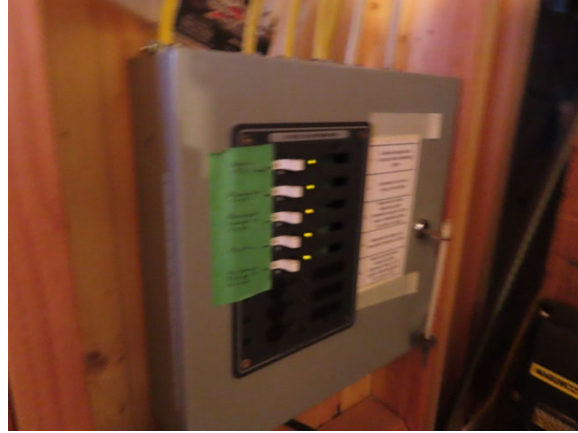
Low-Voltage Lighting System Switch Panel
