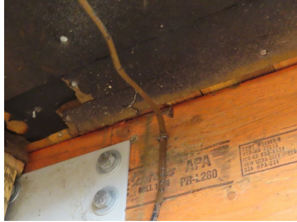
Older Wiring Visible in the Building
