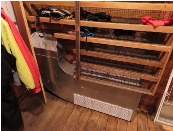
First Floor Furnace Discharge
