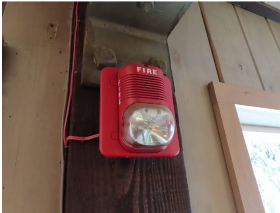
Typical Audio/Visual Alarm
