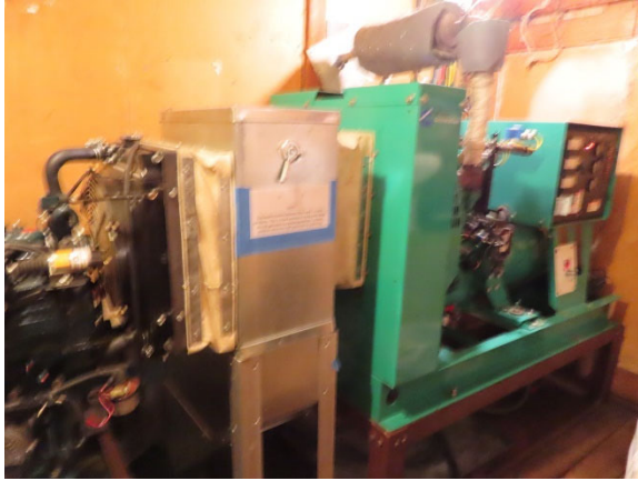
One of Two Generators
