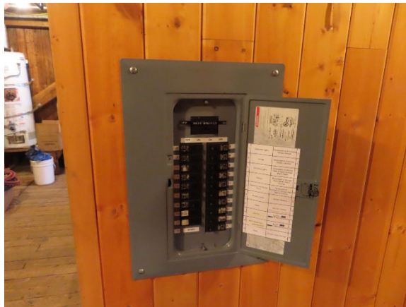
Electrical Service Panel
