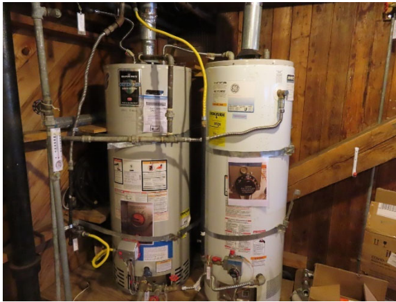
Two Gas Water Heaters
