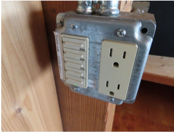
Typical Electrical Outlet and Switch
