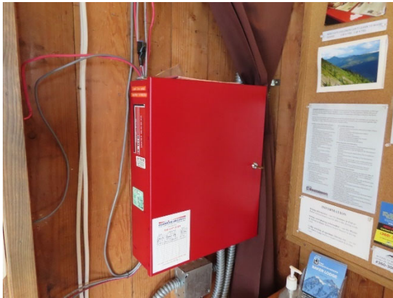
Fire Alarm Control Panel
