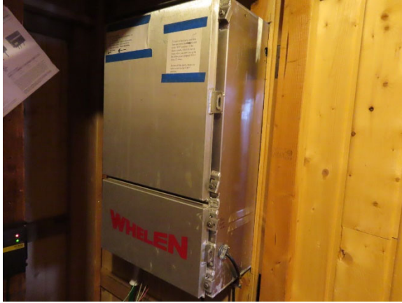
Low-Voltage Lighting System Control Panel
