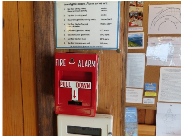
Typical Pull Station
